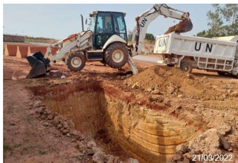
Figure 2. Backhoe Loader for Digging a Septic Tank Immersion Hole in the M'Poko Green Field
