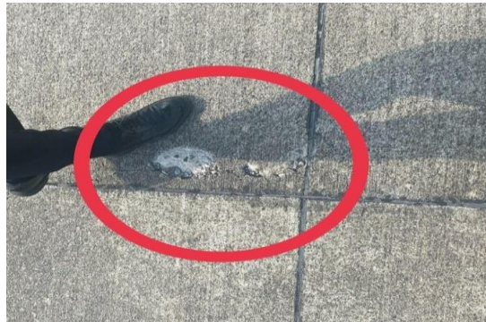
Figure 2. Taxiway Runway Damage Source: Research Documentation
