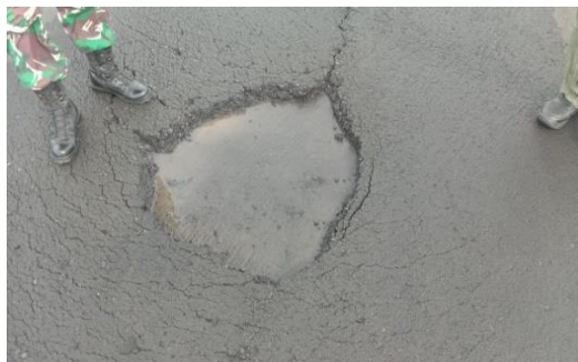
Figure 1. Apron Base Damage
